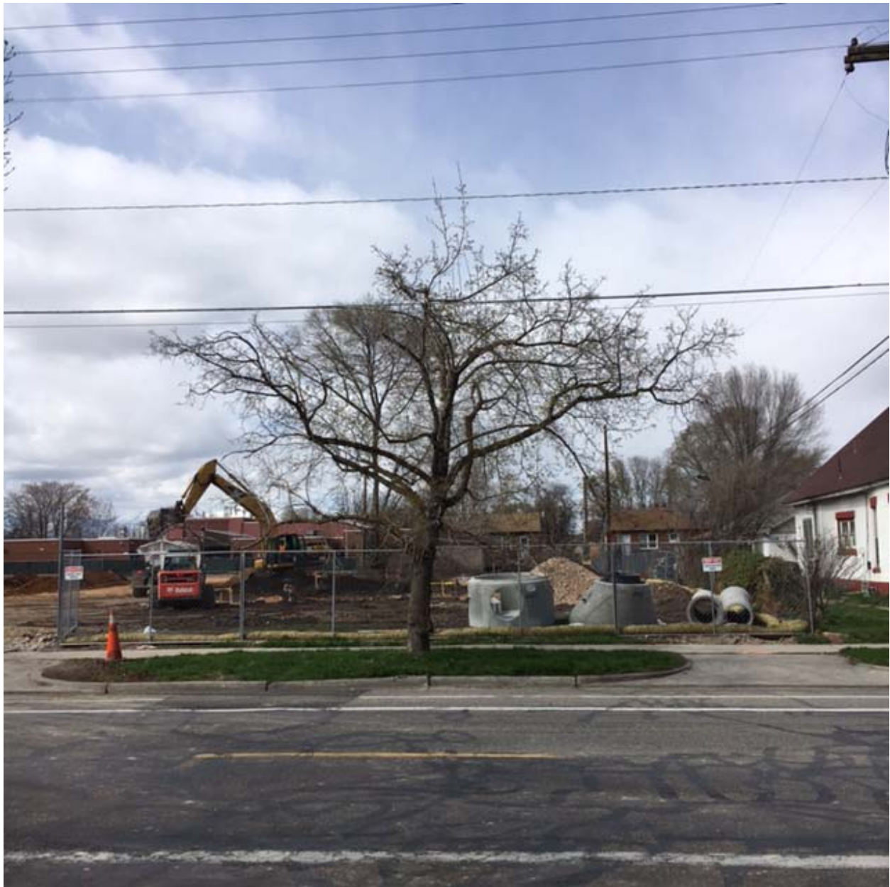
This photograph is looking west from 300 East. One residential structure was demolished where the concrete piping is being stored. Construction on the school can be seen on the left side of the photograph.
