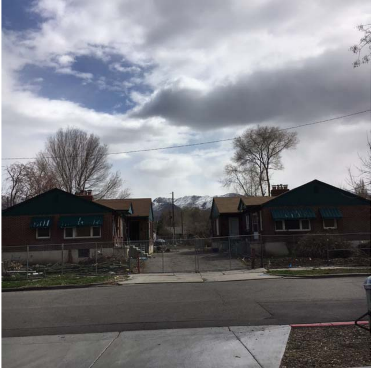
This photograph is looking east on Roberta Street at 2 existing duplexes that are being prepared for demolition. The structures have been demolished since this photograph was taken.
